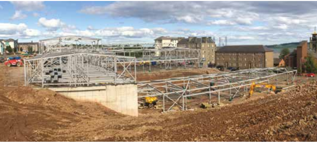
Photo above shows that the main structural steelwork is well progressed, some of which is sitting on substantial reinforced concrete retaining walls constructed by Kilmac.
